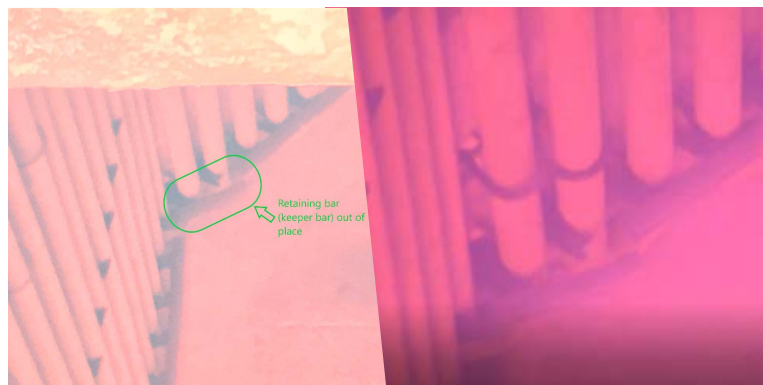
1. Retaining bar out of place
